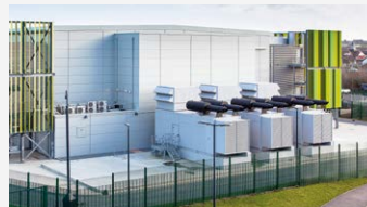
Longcross Park data centre design, delivery and commissioning of MEP infrastructure
