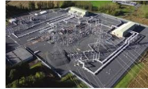
SSE & Scottish Power Earthing solutions across network of substations
